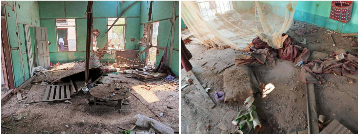
Figure 6: UGC reportedly from the Seik Khun incident demonstrates damage to the inside of a building [22.558029, 95.583815], tea tables and robes are observed among the debris (Source: Karen People's Voice via Facebook).
