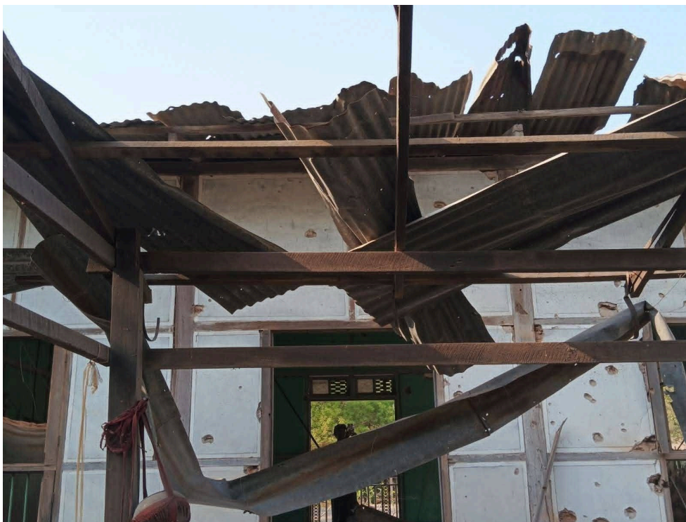
Figure 5: Myanmar Witness analysed the roofing of the external area at [22.557952, 95.583810], which shows indications of a potential aerial attack, due to the inversion of the roofing structure. (Source: redacted).
